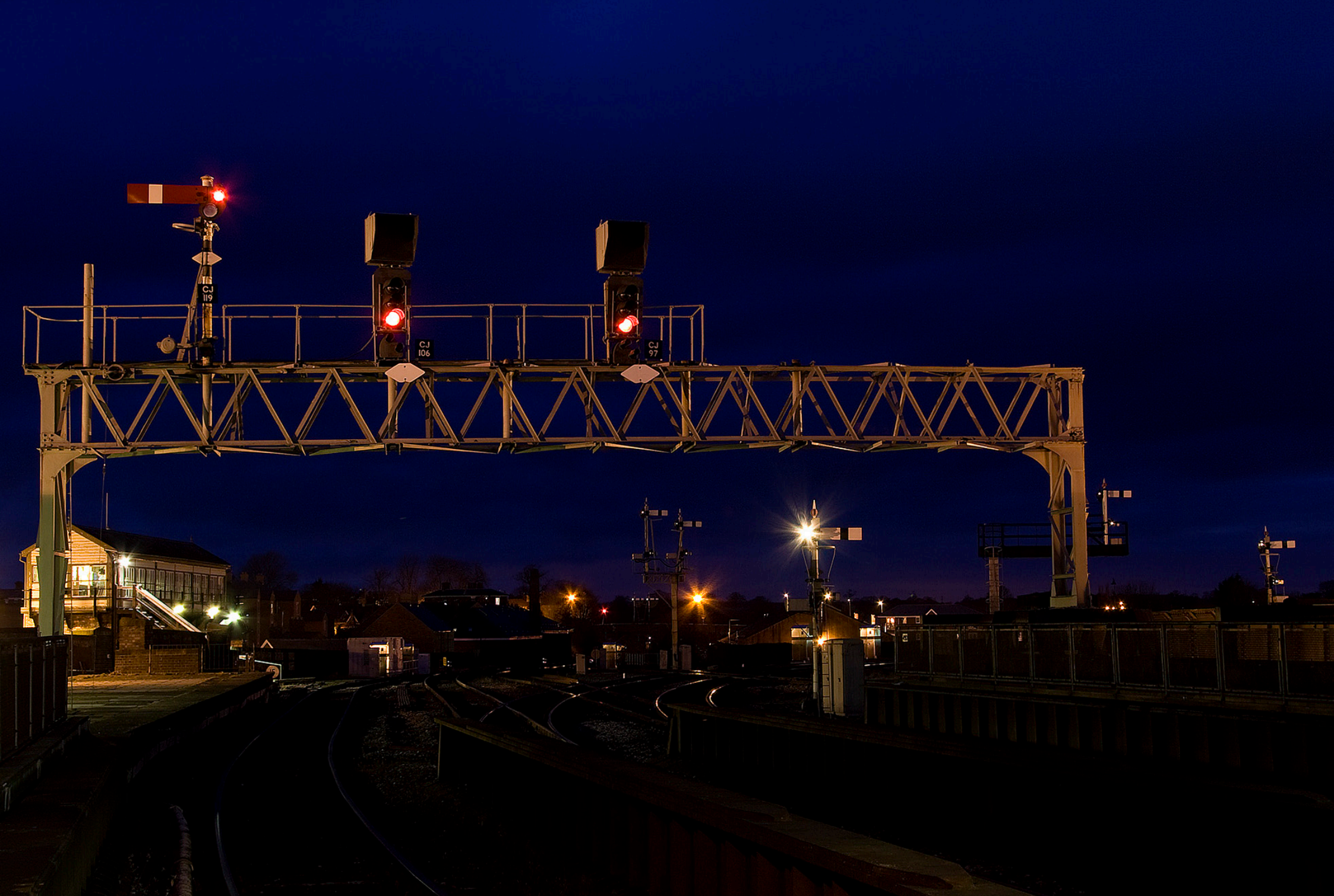
Semaphore signals are slowly disappearing from the rail network, however one location which still has plenty is Shrewsbury, several of which can be seen in this night time shot taken from the north end of the station. Richard Hargreaves
