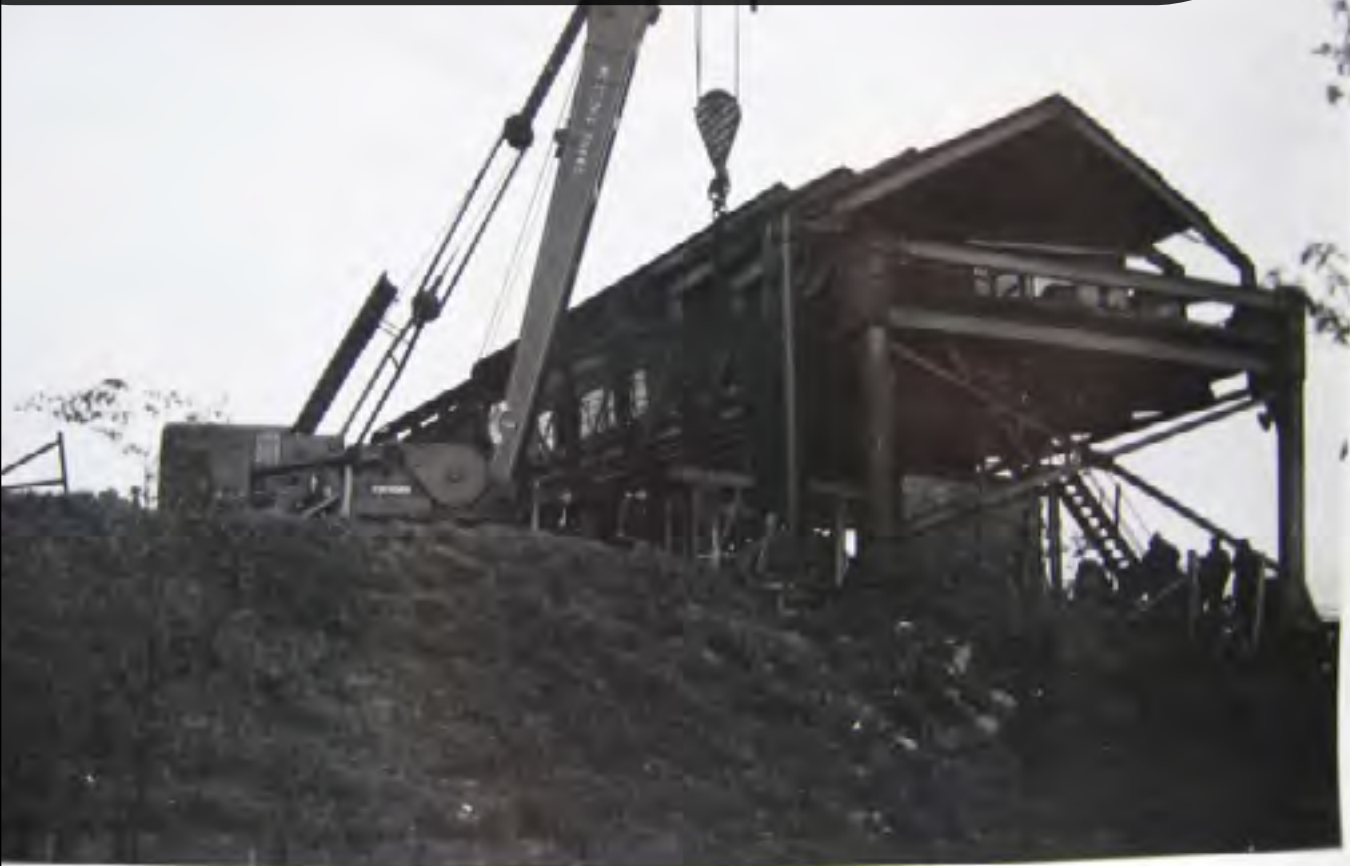
On May 10th 1965, one of the signal boxes at Clapham Junction partially collapsed because of rust in the steelwork. Recovery work is seen in this photo. John Balaam
