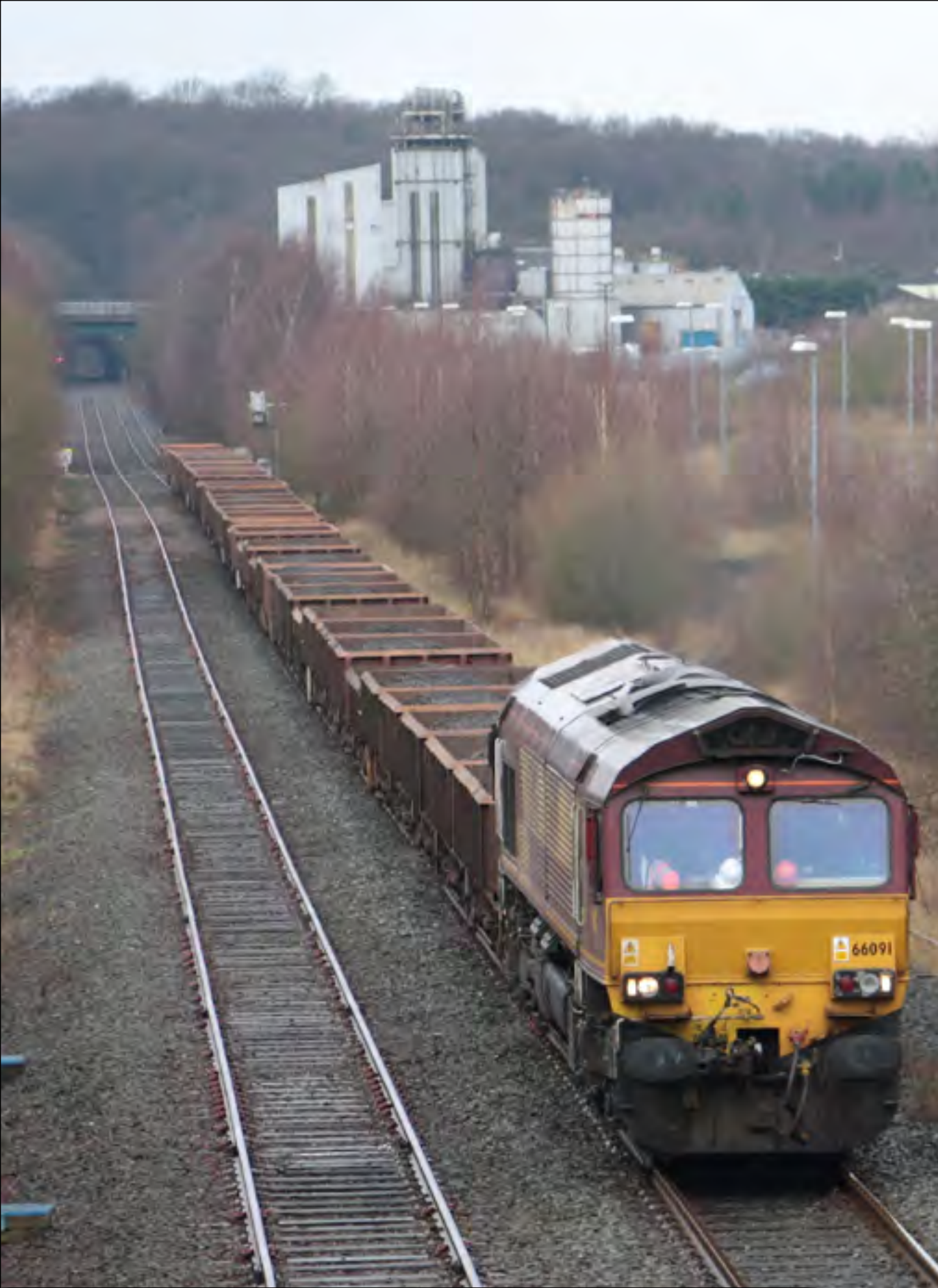
Class 66 091 working the 6B03 Burton's Birmingham Curve Junction - Toton with spent ballast, passes Moira on January 31st. One of several workings during an engineering possession of the Derby to Tamworth line. Stuart Hillis
